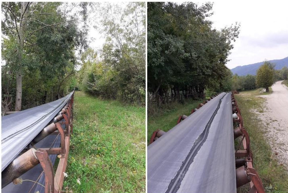
Figure 8. Vegetation obstructing ground visibility
