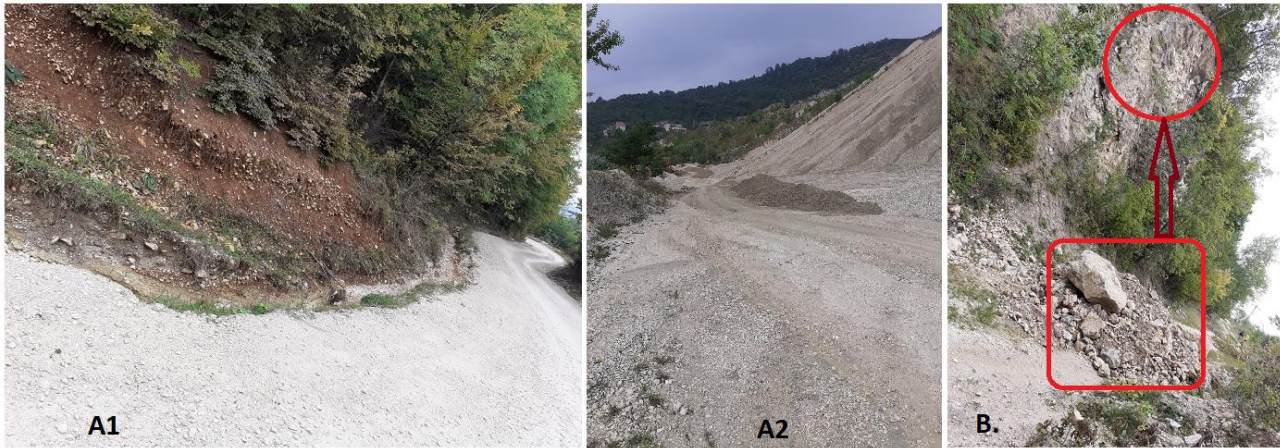
Figure 5. A1 and A2 Access roads affected by precipitation; B. Access Road blocked by dislodged rocks from the slope
