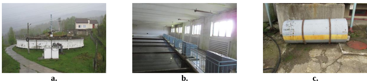
Figure 6. Arrangements and materials within the station: a. Horizontal radial decanter; b. Filter room; c. Tank with liquid chlorine [1]
