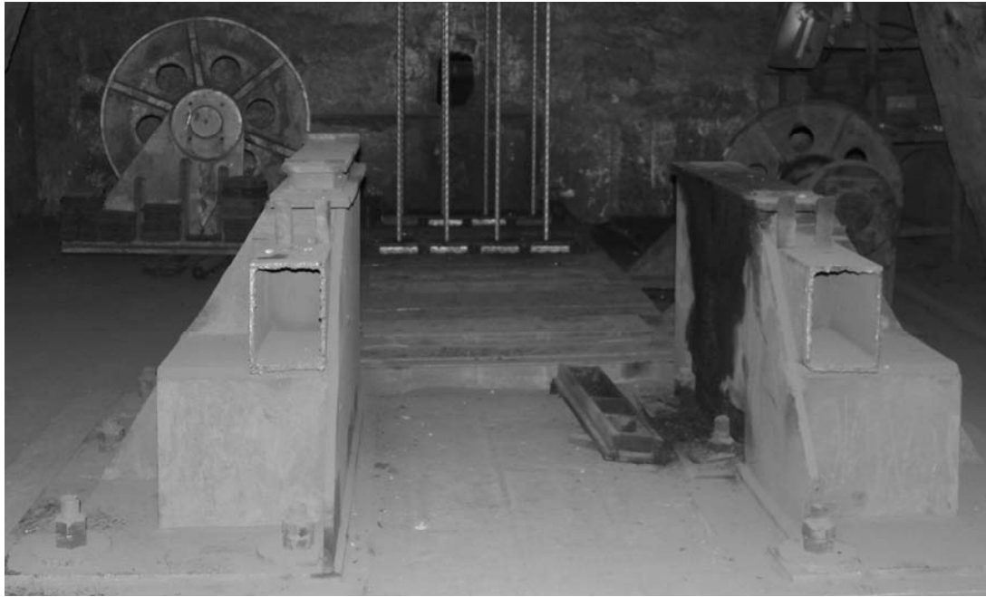
Fig. 3 Cable deviation rolls existing at level 57 of No. 2 Shaft
