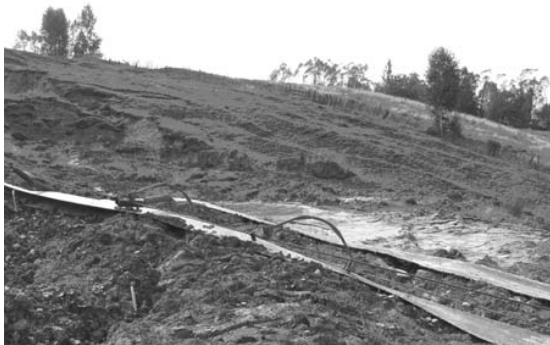
Fig. 7 Discharge phenomena and slope ruptures
