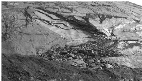
Fig.16. Post failure photograph, May 5, 2014 event
