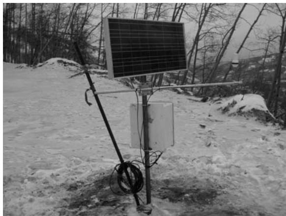
Fig.6. Remotely monitored vibrating wire piezometer
