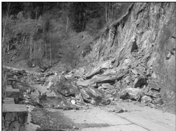
Fig.1 Separation of rock on the road to the dam Gura Apelor
