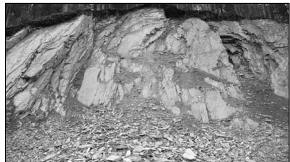
Fig. 7 Ruins and wastelands from altered shale
