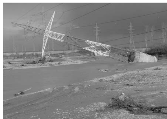
Fig.4 Power Line fell to the ground 220kV Brazi Vest – Fundeni
