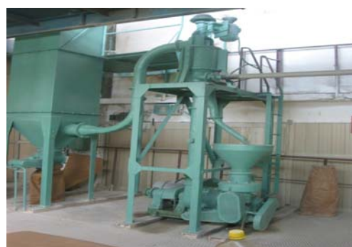
Figure 2 Fine grinding and classing installation
